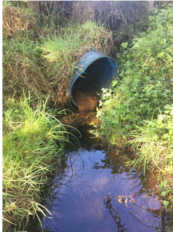
Image 10: Blocked culvert marking the beginning of the permanent stream reach of watercourse three.
